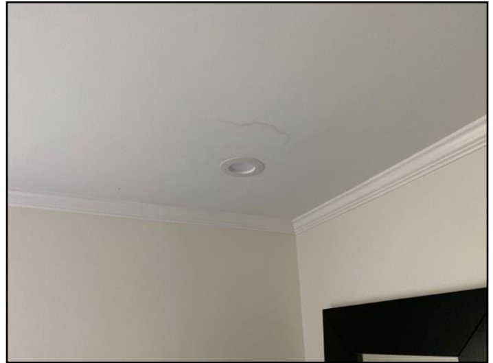
73. Stains noted were dry at inspection.
