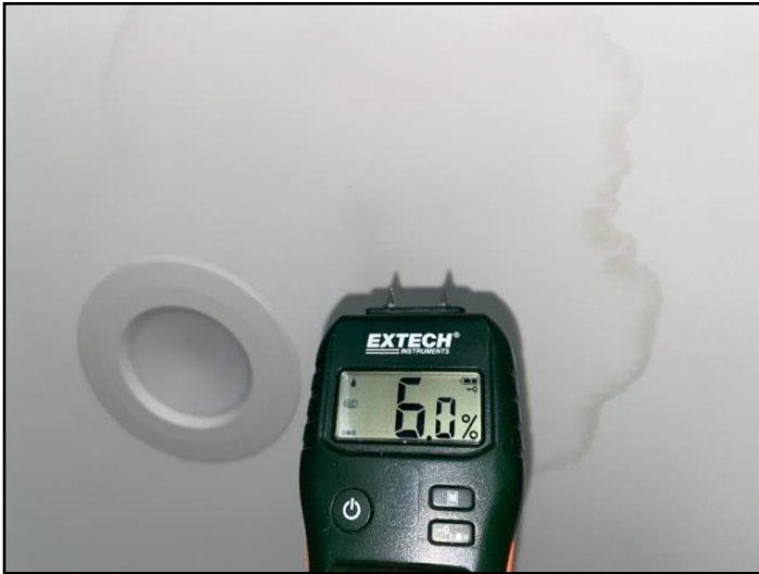
72. Stains noted were dry at inspection.
