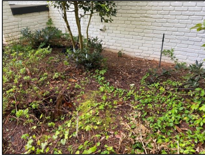
19. Improper Slope or Drainage - Click for DIY...
