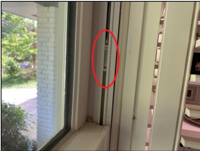
79. Broken Sash Cords/Springs
