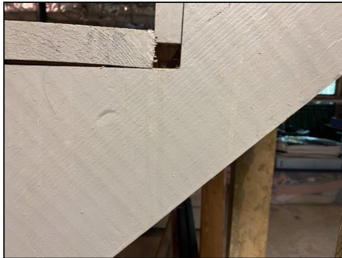
82. Excessive notching of stringers
