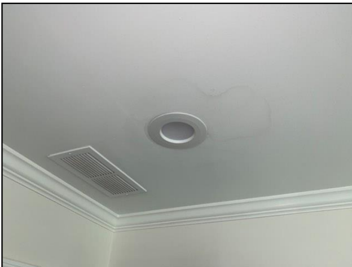
74. Stains noted were dry at inspection.
