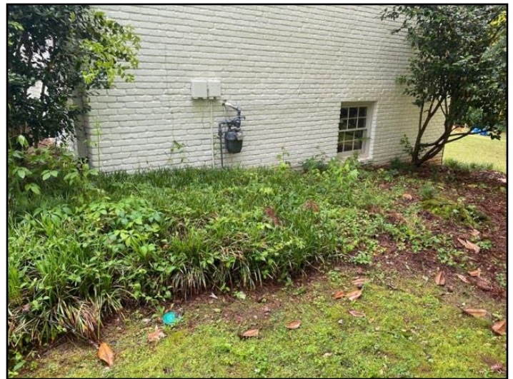
18. Improper Slope or Drainage - Click for DIY...
