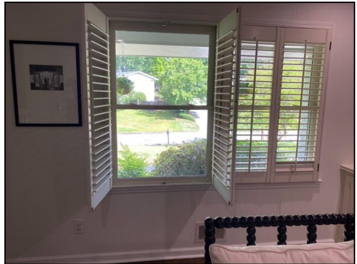
80. Broken Sash Cords/Springs
