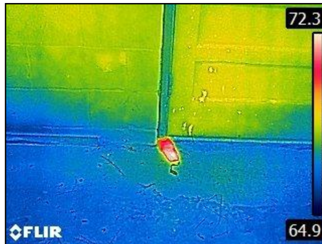
86. Dampness on floor or walls
