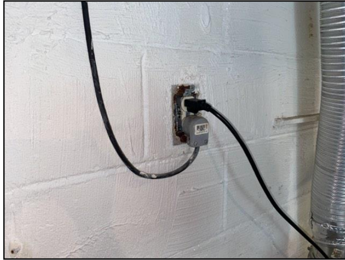
32. Loose, missing, broken cover plate
