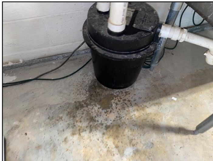
68. Solid waste pump (ejector pump)
