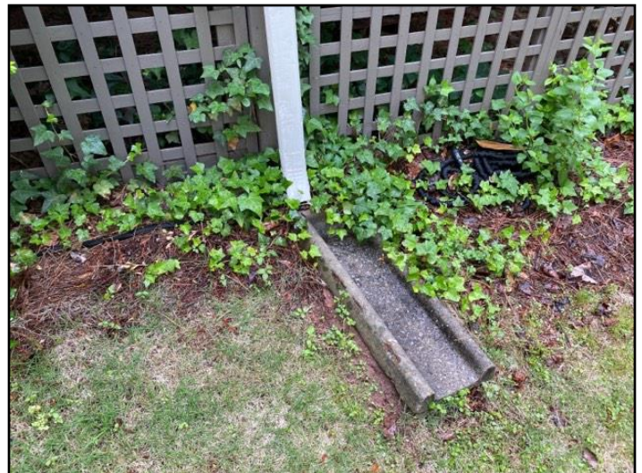
9. Discharges Too Close to the Building
