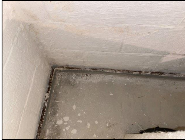
90. Floor patched or Trough at floor perimeter
