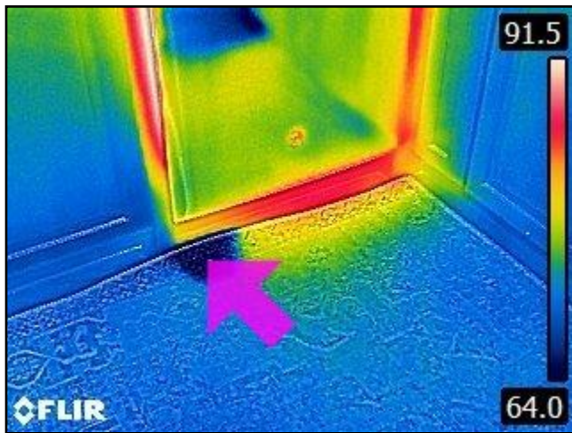
69. Anomaly Noted with Thermal Imaging Scan
