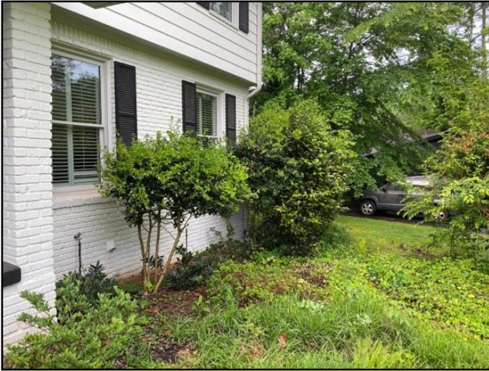
20. Trees or Shrubs too close to building
