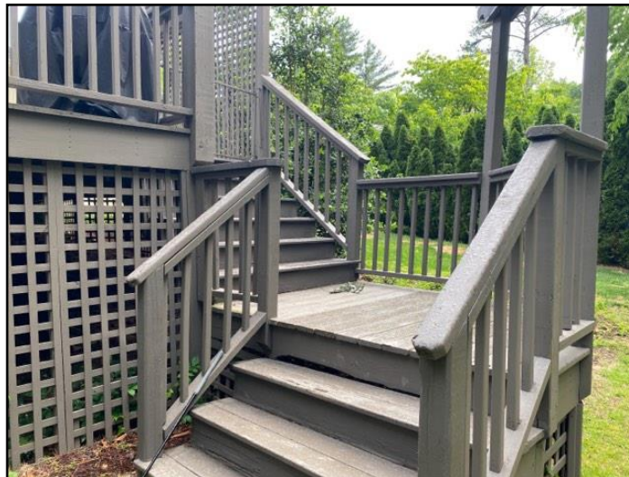
13. Graspable Handrail Missing
