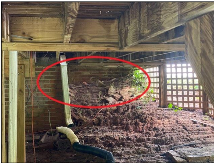
17. Improper Slope or Drainage - Click for DIY...
