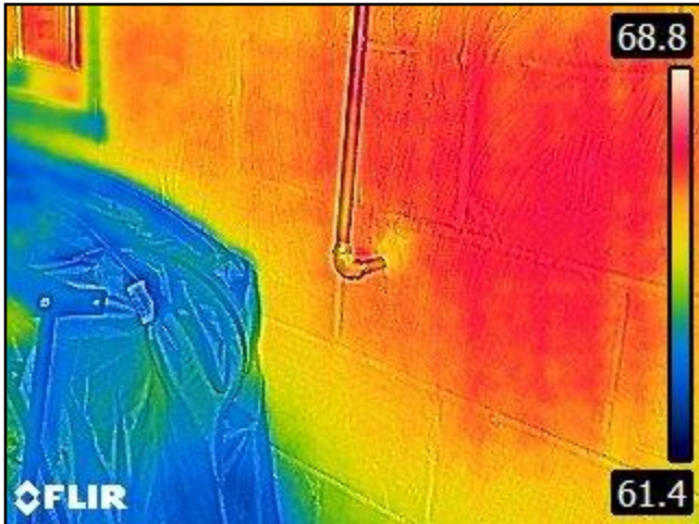
121. Plumbing Fixture/Penetration: No issues
