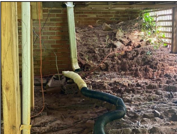
8. Discharges Too Close to the Building
