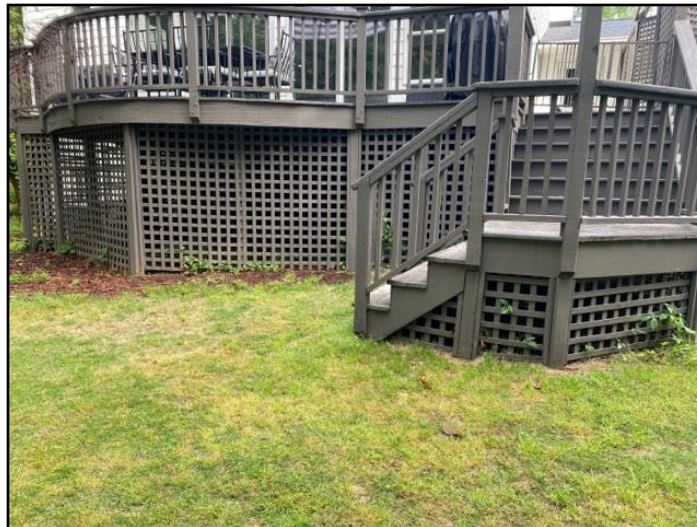
23. Poor access under steps, deck, porch
