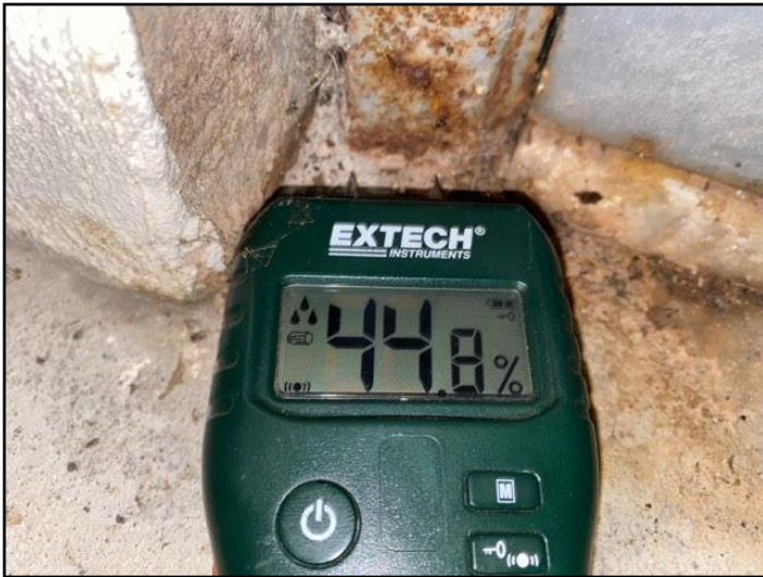
84. Dampness on floor or walls
