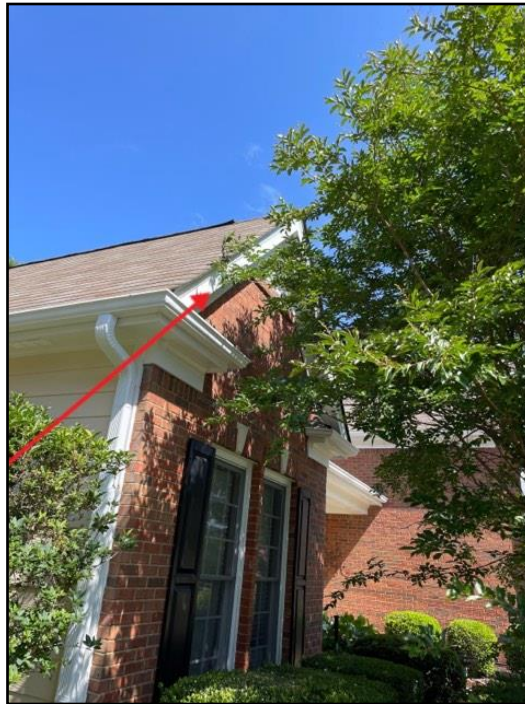
16. Trees or Shrubs too close to building
