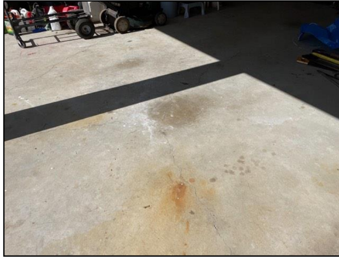
20. Cracks in Floor
