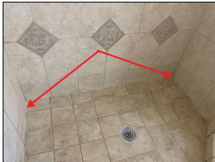
45. Caulking/Grout missing and or deteriorated...
