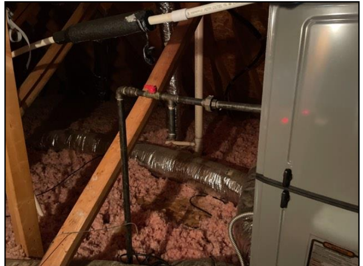
28. No drip leg (sediment trap, dirt pocket)
