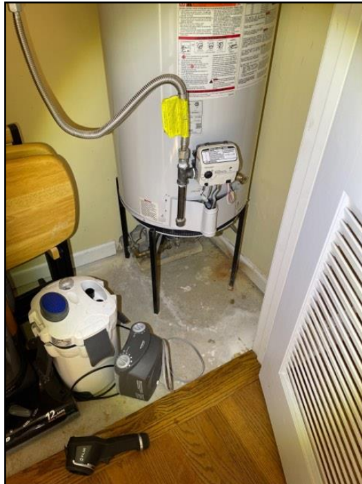
43. Drain pan missing
