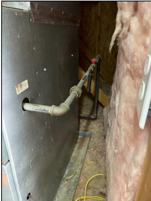
27. No drip leg (sediment trap, dirt pocket)
