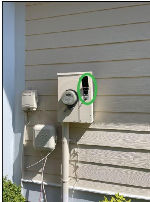
24. Breakers - exterior wall
