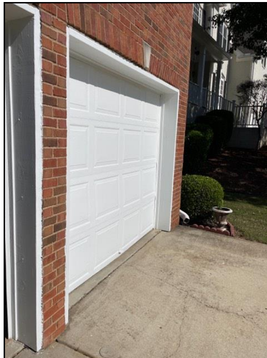
19. Vehicle Door is Dented/Damaged
