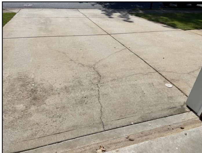
17. Cracked or Damaged Surfaces
