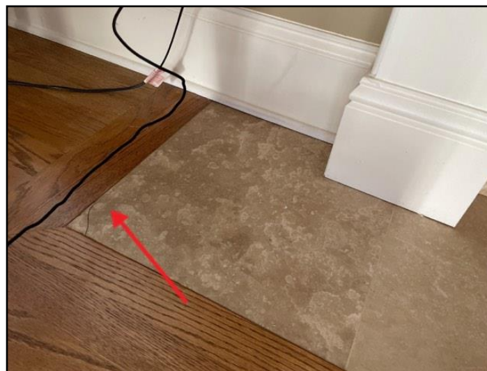
29. Gaps or cracks
