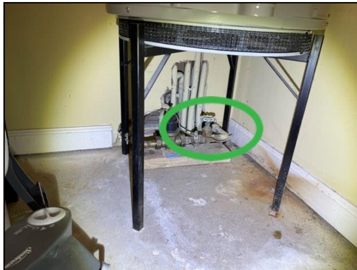
48. Near water heater
