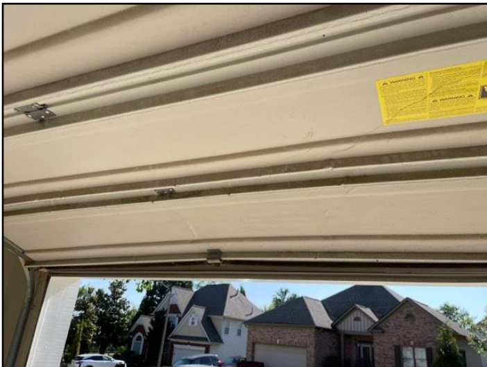
18. Vehicle Door is Dented/Damaged
