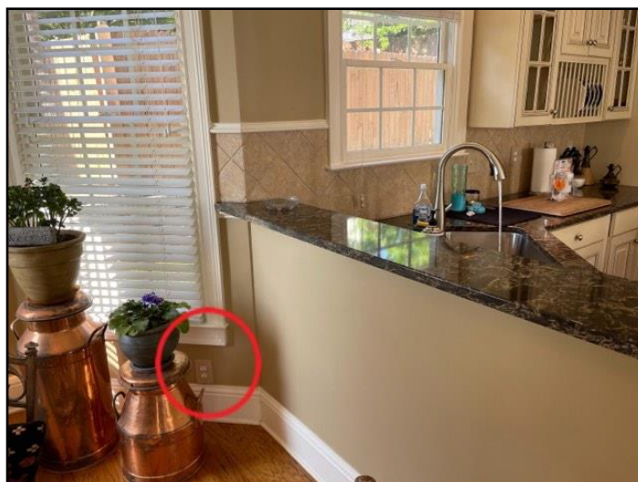
22. No GFCI/GFI (Ground Fault Circuit...)
