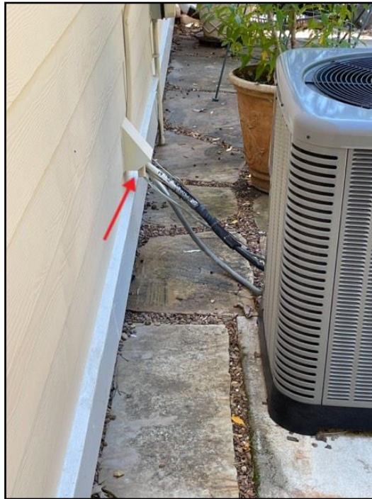
38. Improper Discharge Point
