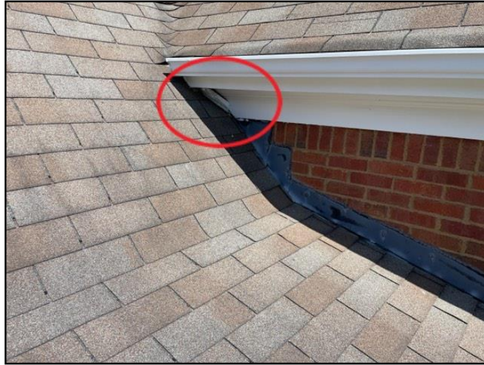
15. Loose or missing pieces
