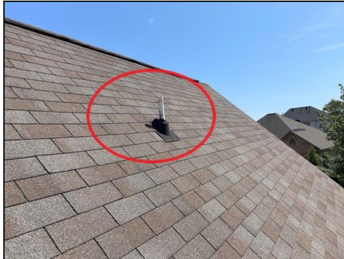
9. Damage, loose, rusted or missing
